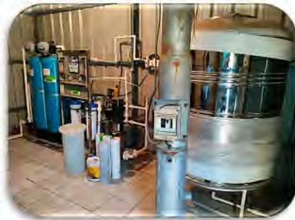
Project- Social Welfare RO Drinking water facility, Taloja
